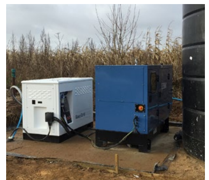
System: EasyGrid 10000 with a 8kW ground mounted solar array and 22 kVA SDMO generator.
